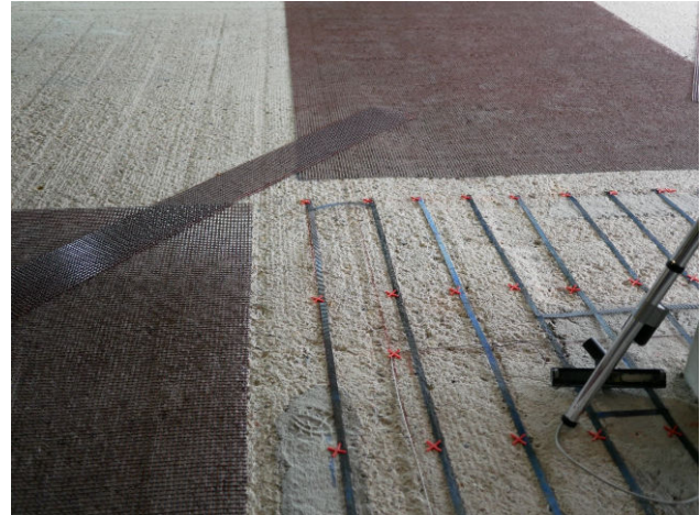
Carbon scrims on bare concrete slabs, with anode strips surrounding the supports to protect against cathodic corrosion (on the right)
